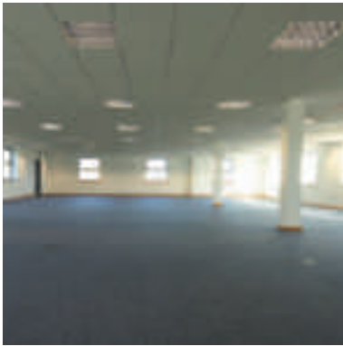
Suspended ceilings with recessed lighting.
