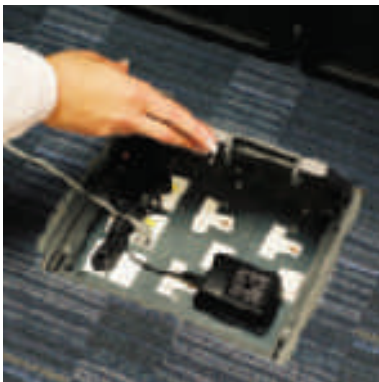
Fully raised access floors.
