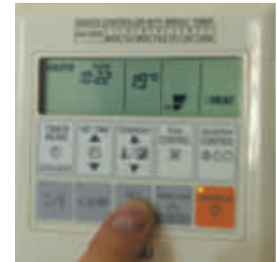
Air conditioning (comfort conditioning) as standard.
