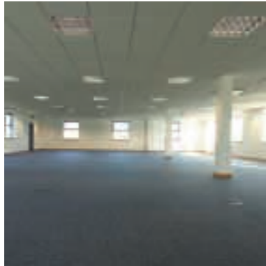
Suspended ceilings with recessed lighting.
